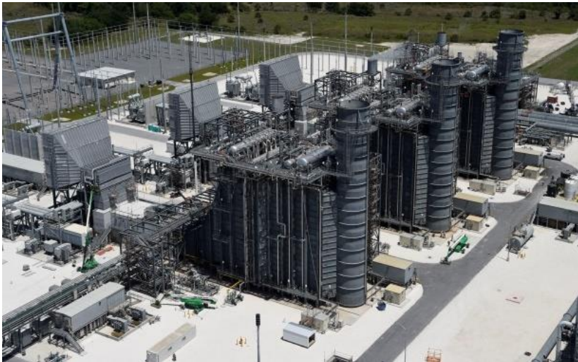
FPL's Okeechobee Clean Energy Center COD March 2019
